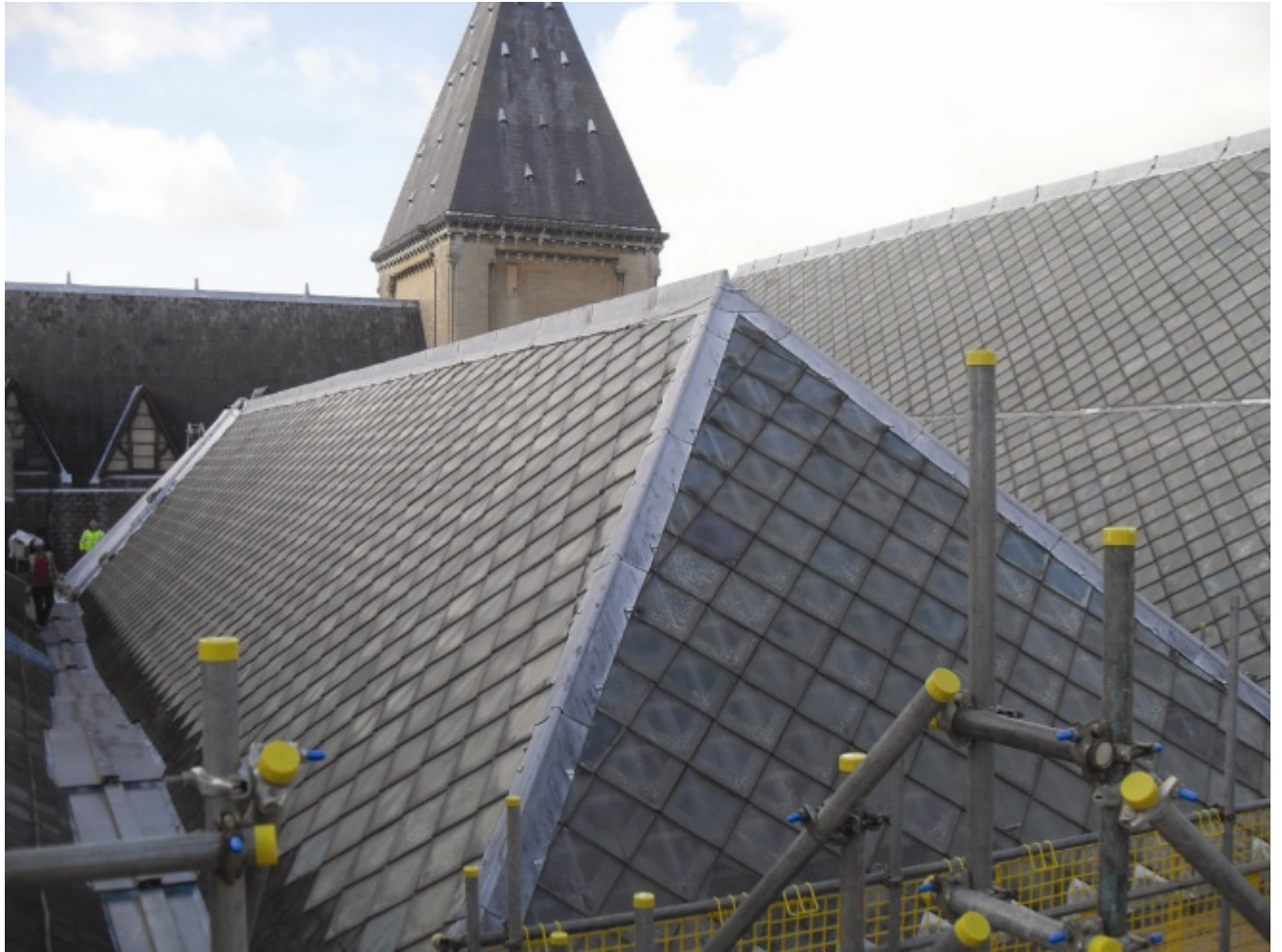
Before restoration the roof leaked and was dirty
